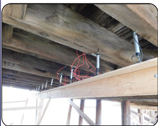
Image 26. Load Testing Sensors Measuring Displacement on US 36 over Vega Creek in Washington County
